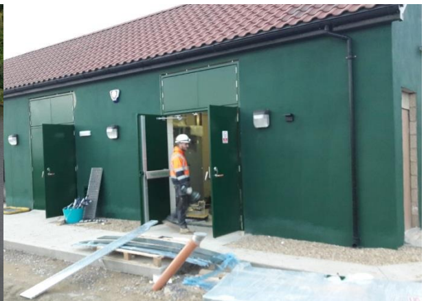
Wind Farm Control Building
